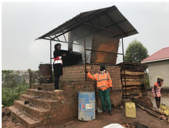
Water for People's newly constructed carbonization unit at Lubigi. (source: presentation by Ms. Lugali)
