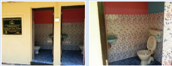
Sanitation facility at St. Bartholomew's High School, Chorao Island, North Goa, India (Photo credit: TERI, Goa).
