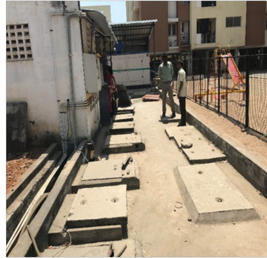
Figure 7: Small Scale STP installed in a gated colony comprising 80 residential units in ward 20 (Kripa/Eawag,2019)
