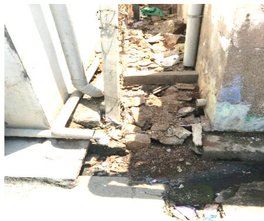
Figure 1: Greywater discharged into open drains where sewer network is present (Harsh/GIZ,2019)
