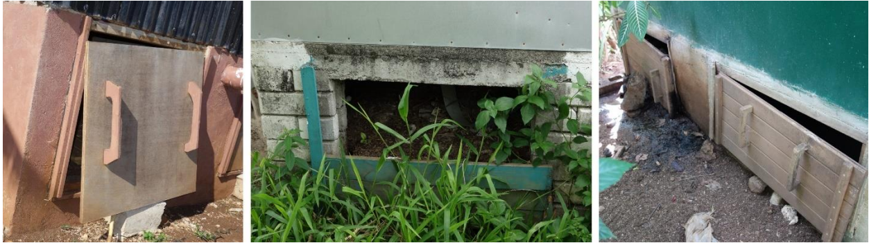
Figure 7: Defect vault doors of Composting Toilets in Vanuatu.
