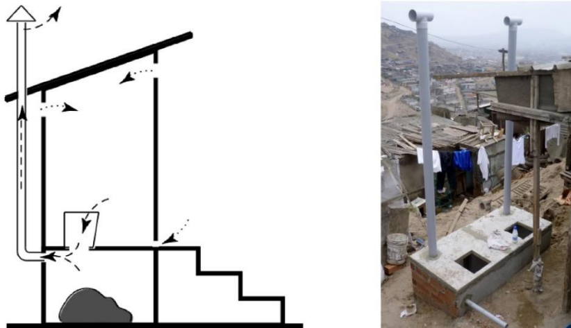
Figure 11: Air flow of natural ventilation system of a UDDT (left) (WiSDOM, 2016, p. 16, adapted); Construction of double dehydration vaults, each equipped with proper ventilation pipes (right) (Rieck et al., 2012, p. 17, adapted).
