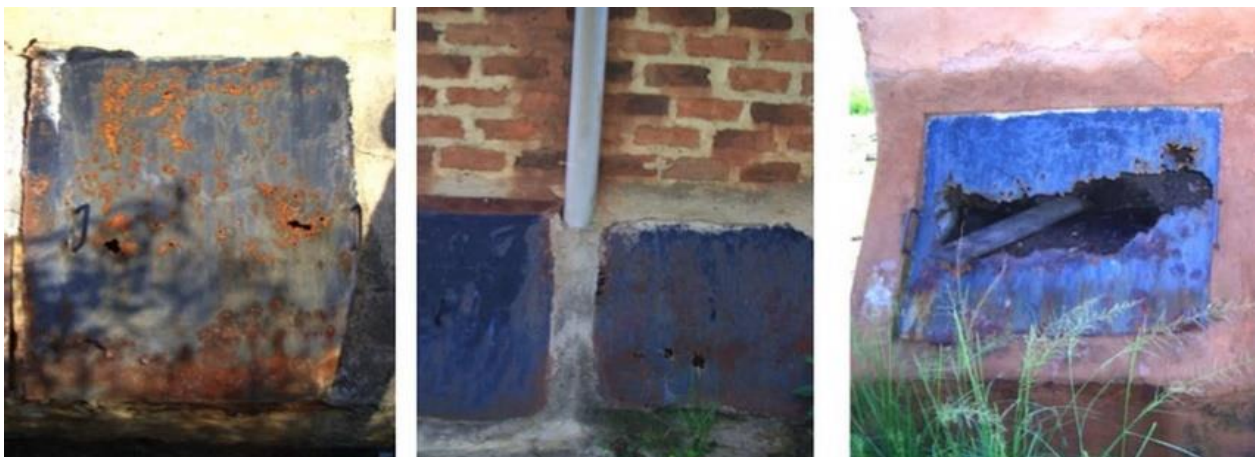
Figure 10: Corroded iron sheets of solar UDDTs (Windberg & Otterpohl, 2016, p. 1266, adapted).
