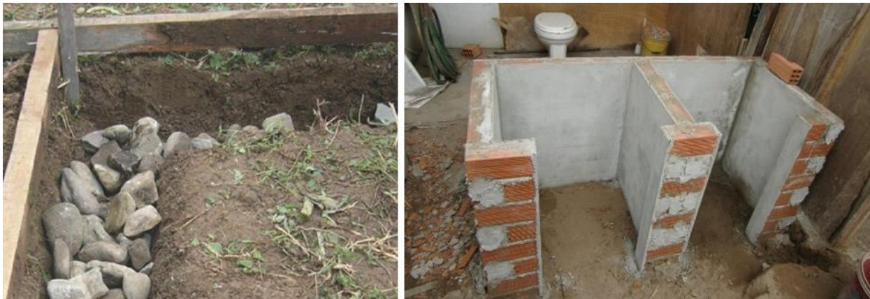
Figure 6: Stone-filled excavation for foundation (left) (WECF, 2015, p. 26, adapted), Vault construction with bricks (right) (Rieck et al., 2012, p. 17, adapted).
