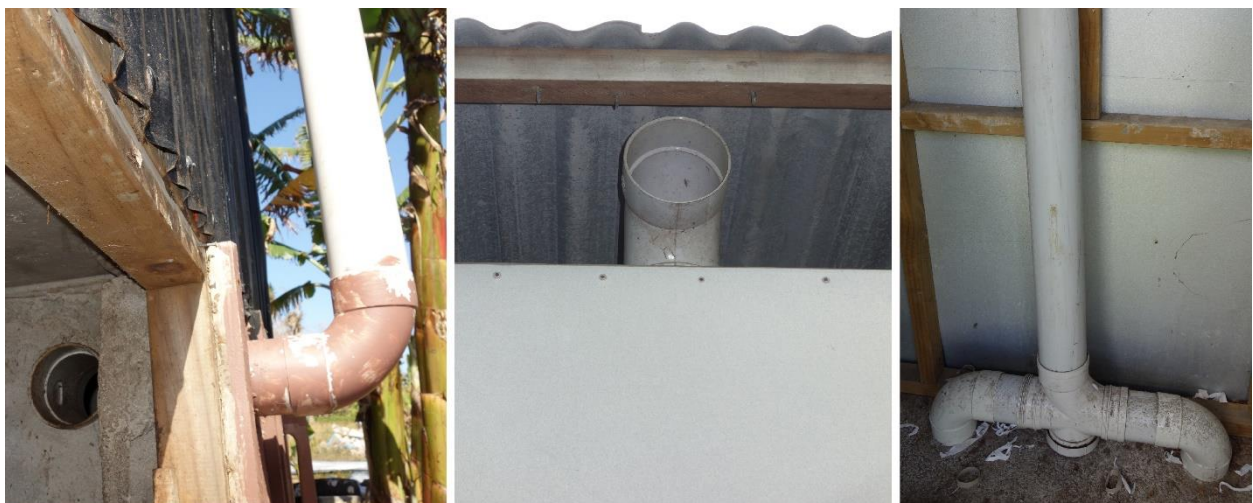
Figure 13: Examples of poorly designed ventilation pipes of Composting Toilets in Vanuatu (left & right: Only one pipe with 90° corners for both vaults; centre: Ventilation pipe with 90° corner does not extend above the roof of the superstructure).
