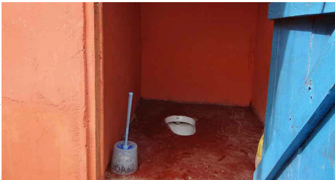
Picture 6: Dry toilet constructed as part of the UBSUP programme in Kenya
