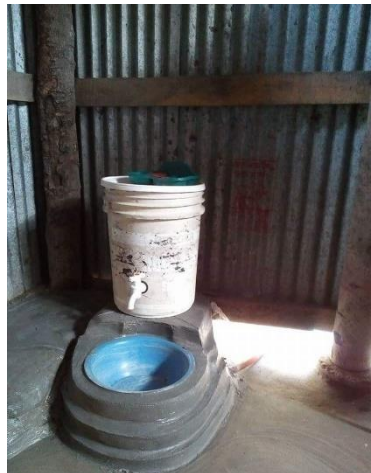
Used paint container with tap and installed inside the kitchen along with plastic bowl for basin
