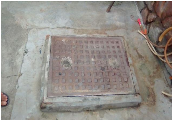
Figure 3: Septic Tank connected to sewer line in Ward no. 4 (Niharika/CSE, 2020)
