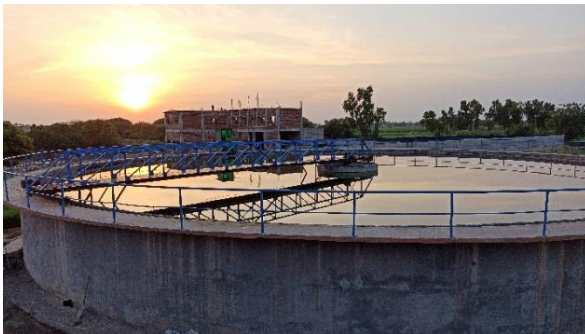
STP at Kelniyan
