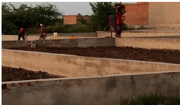
Sludge drying beds at Kelniyan STP
