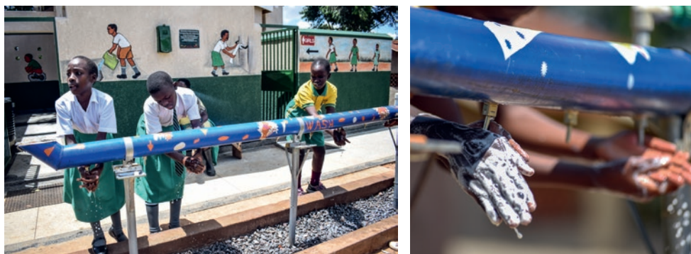
Figure 3: WASHaLOT 3.0 group handwashing facilities installed at St. Paul Ggaba demonstration primary school, Kampala.
