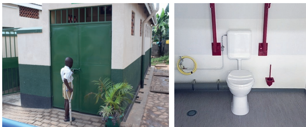
Figure 2: Whilst all students at St Peter's benefit from the new and well-equipped sanitation facilities, school life has become a great deal easier for pupils with disabilities.
