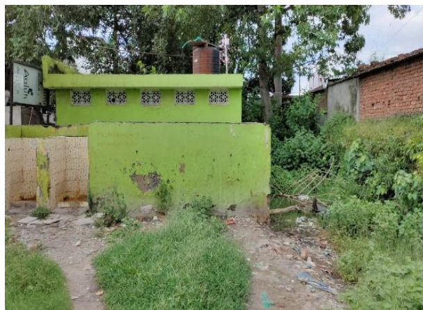
Figure 3: Fully lined tank connected to open drain in Forsytganz Public Toilet (Saiyami/CSE, 2020).
