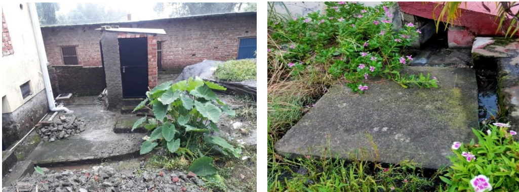
Figure 2: Fully Lined Tank connected to open drain in a household (Saiyami/CSE, 2020).
