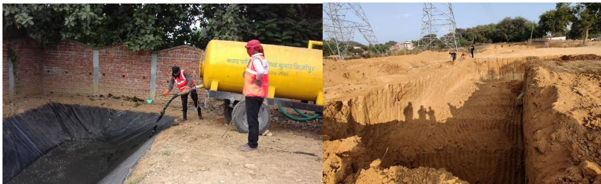
Figure 3: Temporary trenching facility (on the left) and Faecal Sludge Treatment Plant (on the right) (Manish/CSE, 2020)
