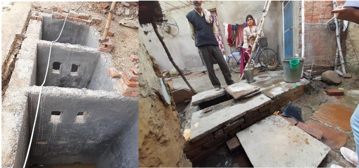
Figure 1: Septic Tank under construction and fully lined tank connected to open drain (Manish/CSE,2020)
