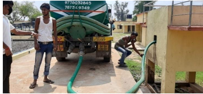
Fig 7: Septage Treatment Plant (Source: CSE, 2020)
