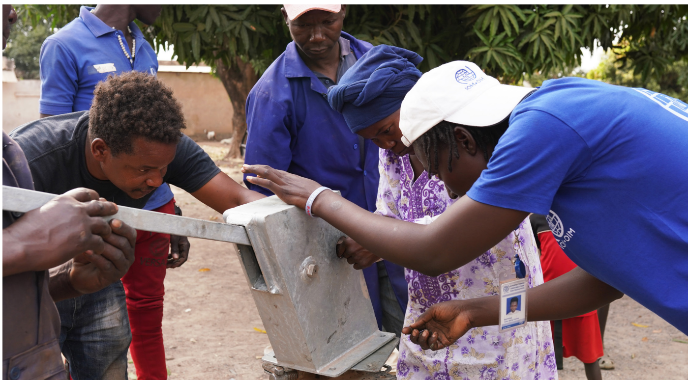
Women and men hand pump mechanics work together to repair a borehole in Wau, Western Bahr el Gazal, South Sudan. ©IOM 2020 / Andreea CÂMPEANU
