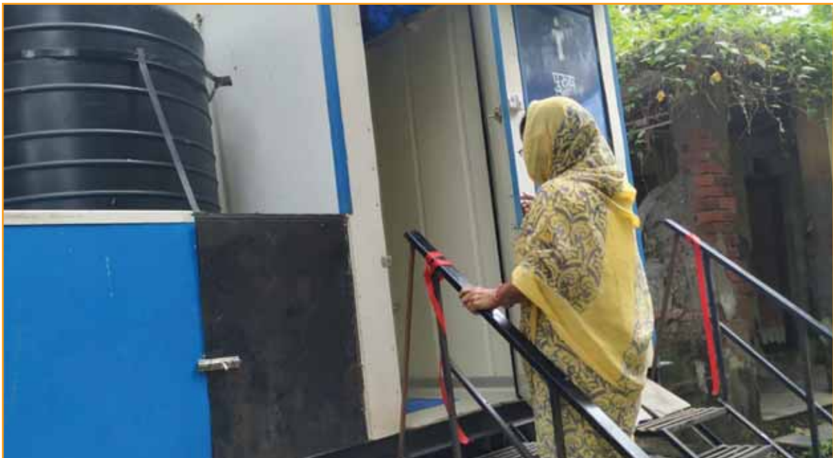
Figure 18: Mobile toilets installed by LIXIL SATO in active partnership with UNICEF Mumbai
