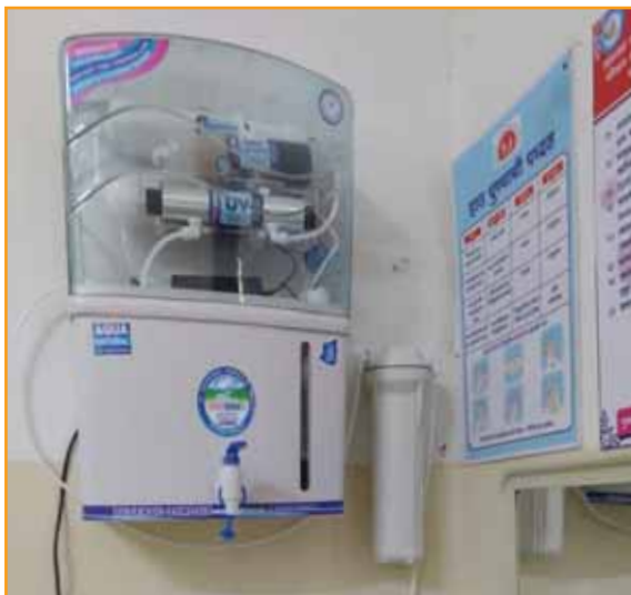
Figure 11: Before and after providing access to better quality of drinking water at the Minatai Thakare Polyclinic, Vadgaon Sheri, Pune
