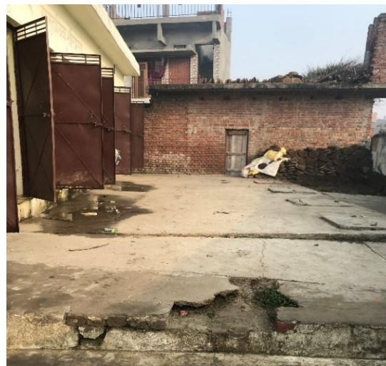
Figure 3: Septic Tank of a Community Toilet at Harijan Basti (Harsh/CSE, 2020)
