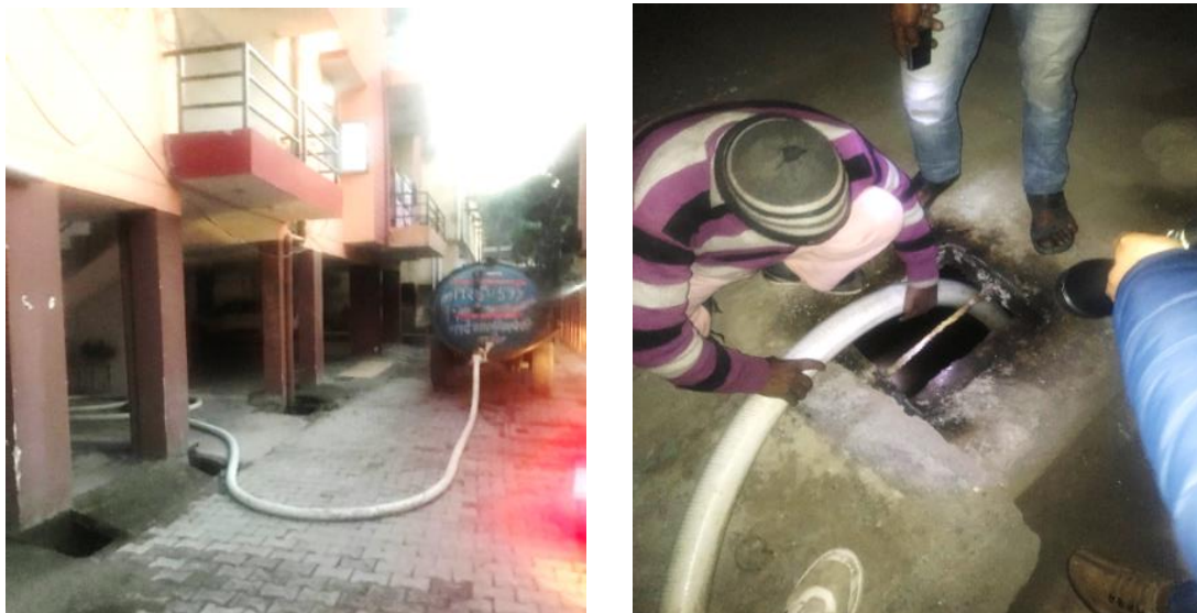
Figure 5: Emptying process captured near Palika Chowk in a common septic tank tank of 8 households. (Harsh/CSE, 2020)
