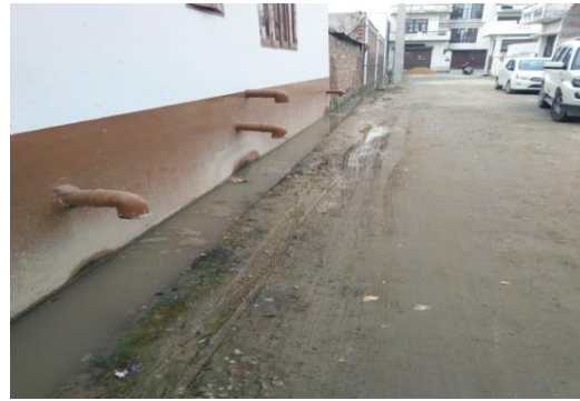
Outlet connected to open Drain
