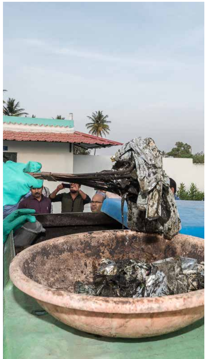
Figure 11 - Efficient removal of solid waste from the feeding tank of the FSTP after design modification of the screens
