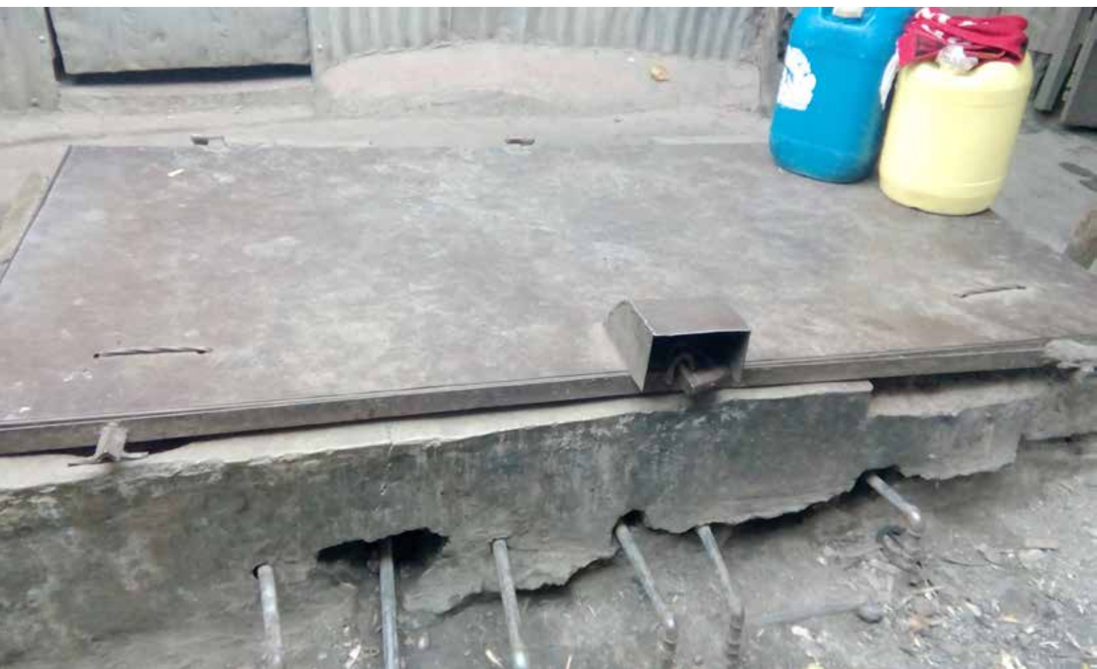
Abandoned chambers in Mukuru in Zone 48.
