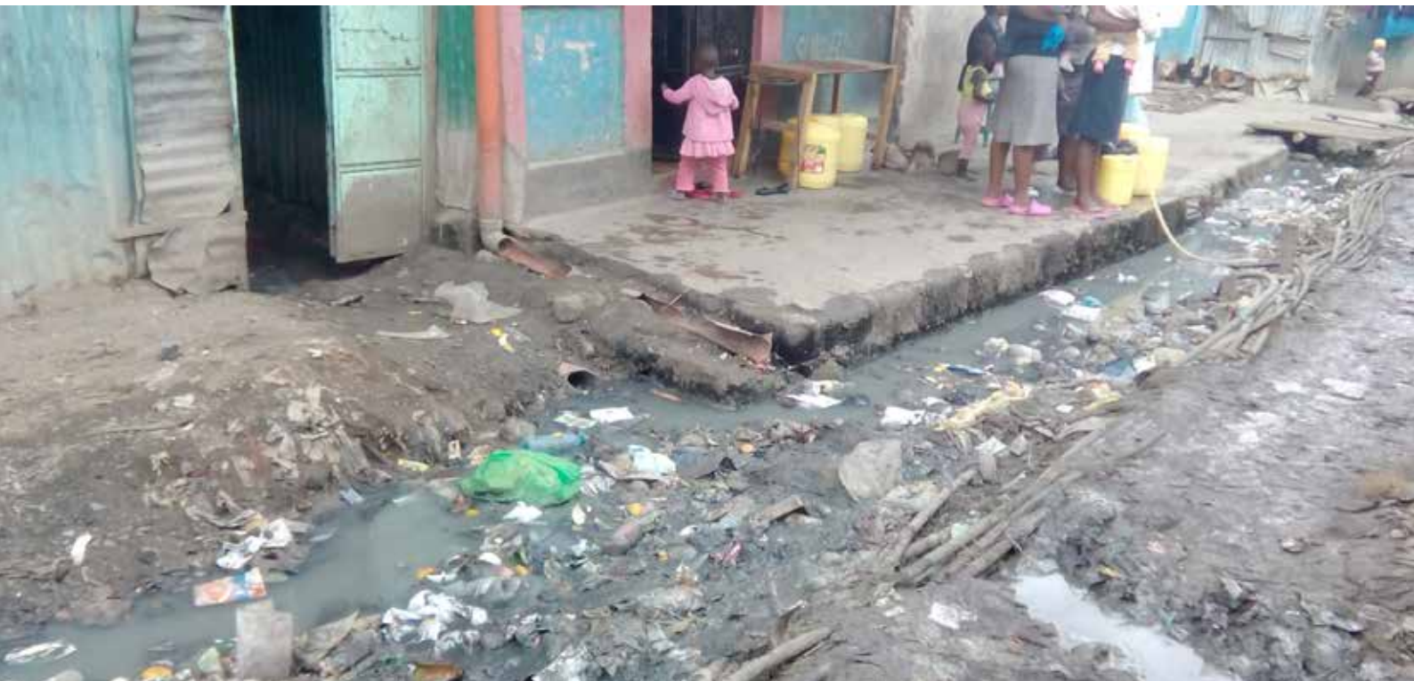
Water pipes running in unsanitary conditions in Moto Moto Village in Mukuru.
