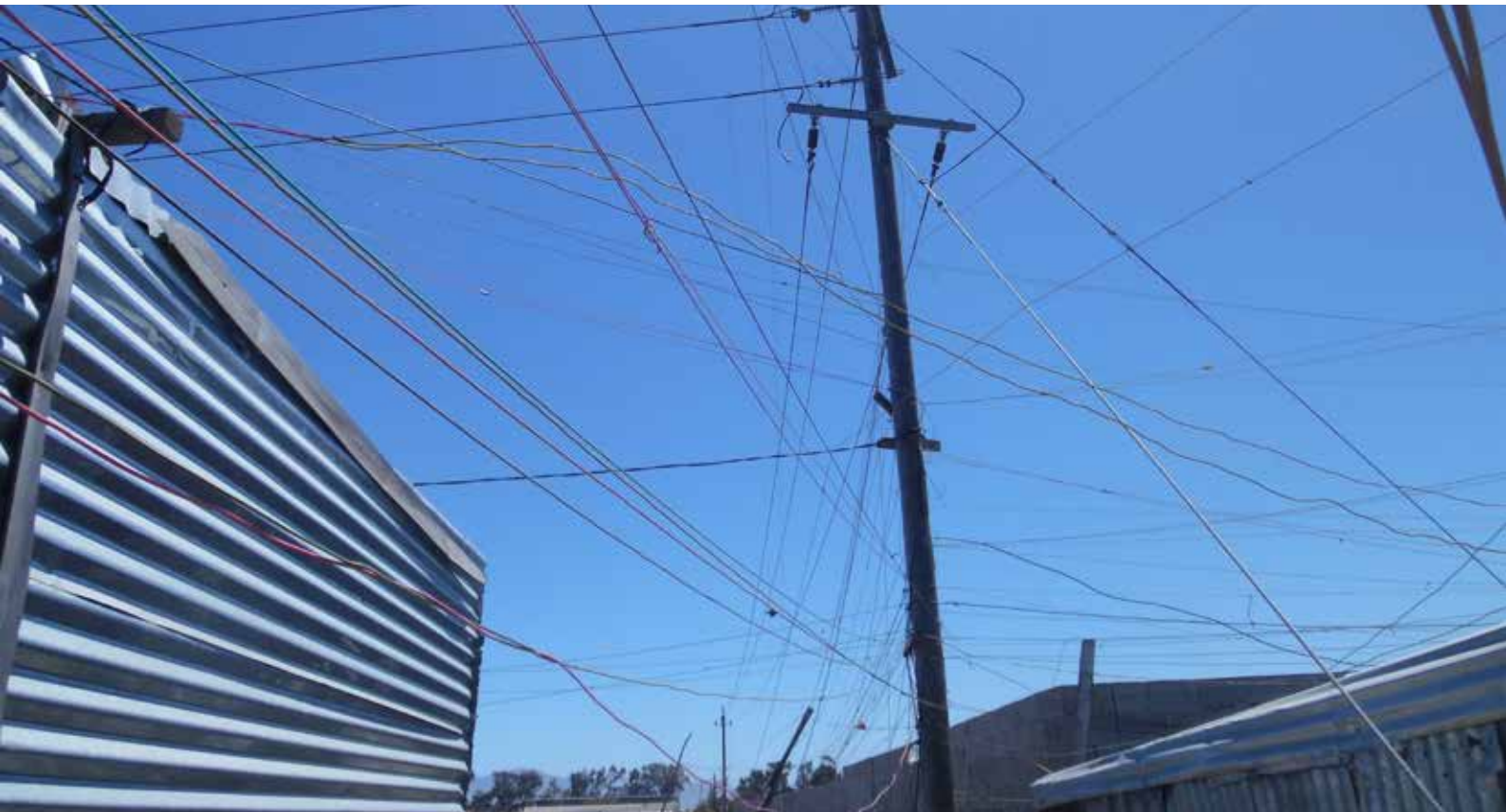
Self made electricity connections, Marikana.
