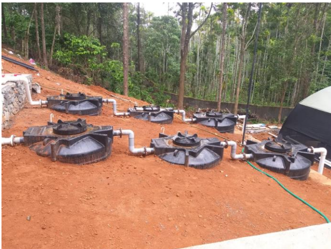
Anaerobic Digesters installed
