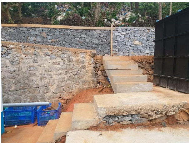
Access to all parts of the FSTP
