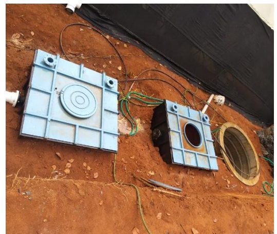
Intermediate collection tanks for partially treated effluent
