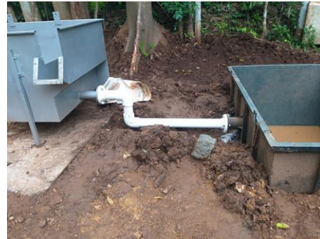
Screen to SST plumbing
