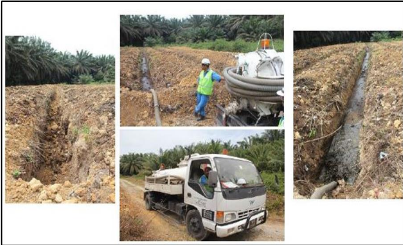
Figure 10 – Deep Row Entrenchment
