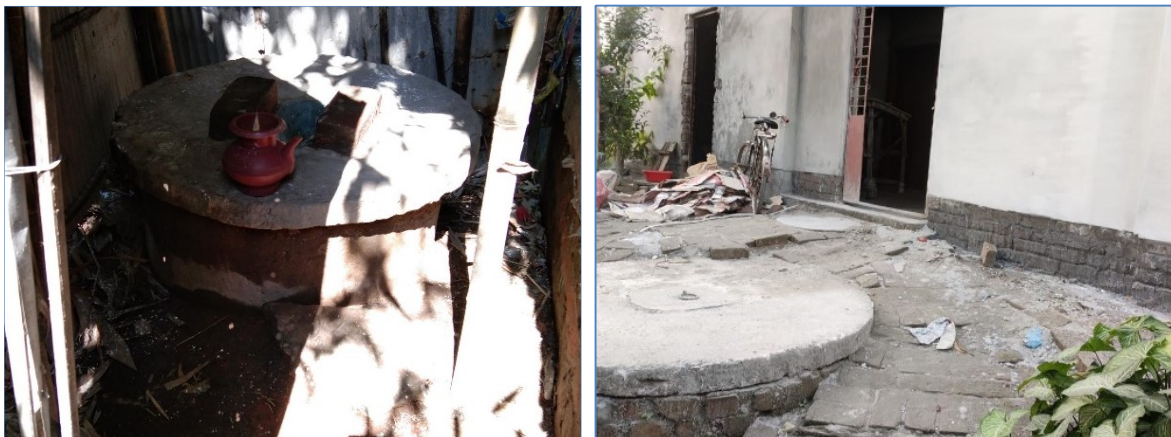
Figure 2: Pit (left) and septic tank with soak pit system (right) (Source: Binte, 2020).
