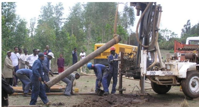
Figure 5: Poor Safety – No Hard Hat – No Clearly Defined Barrier
