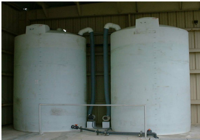
Figure 4 Typical Sodium Hypochlorite Storage Tanks with Hydrogen Dilution Fans
