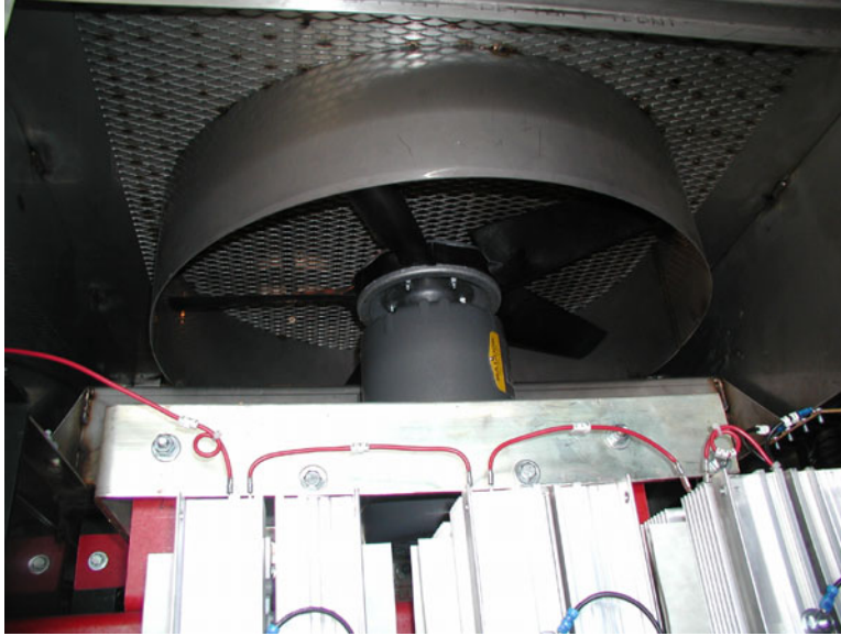
Figure 8 Typical SCR (Thyristor) Rectifier Cooling Fan Arrangement
