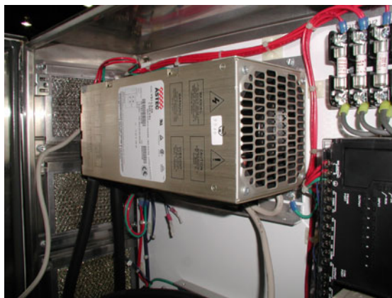
Figure 7 Typical Switching Power Rectifier in Control Panel
