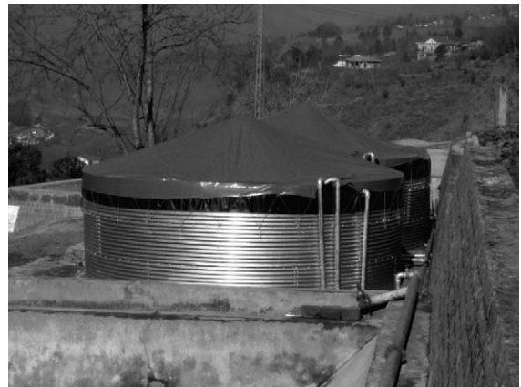
Fig. 2. Batch coagulation tanks used in Gahri Doppata (Pakistan).
