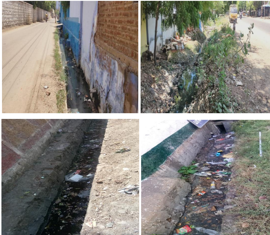
Figure 3: Blockage of open medium sized drains.
