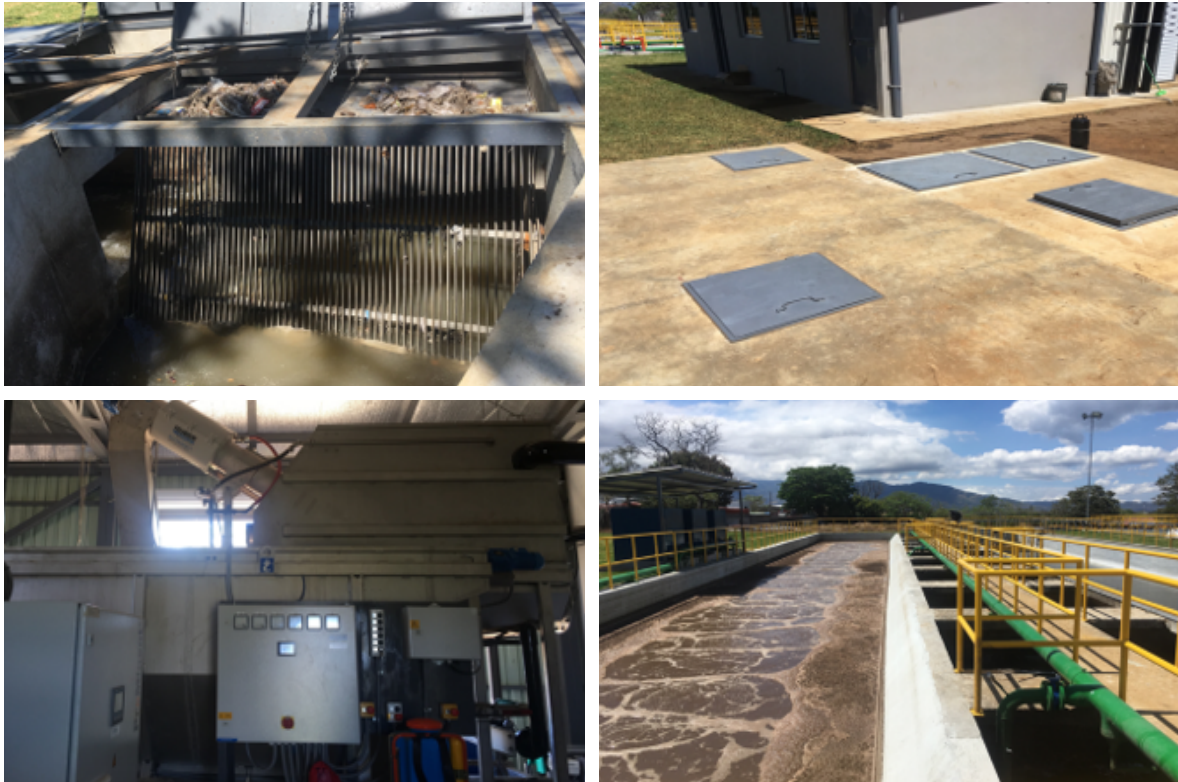
Figure 6: Villa Bonita WWTP. Upper Left: Wastewater Intake. Upper Right: FS Intake. Bottom Left: HUBER Rotamat® Pretreatment Machine. Bottom Right: Aerobic Wastewater Treatment, Primary Sedimentation and Digestion Reactor
