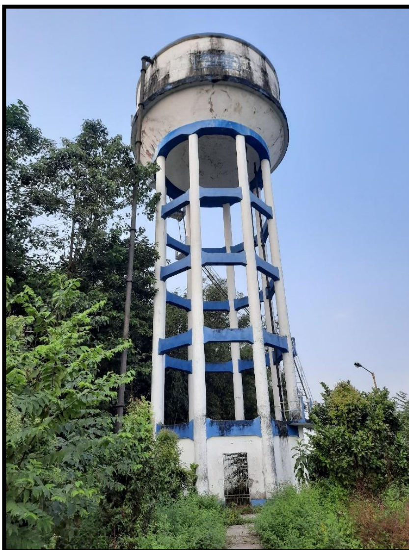
Image 5: OHR at Pump house of Baneshwar Water Supply Scheme, Coochbehar
