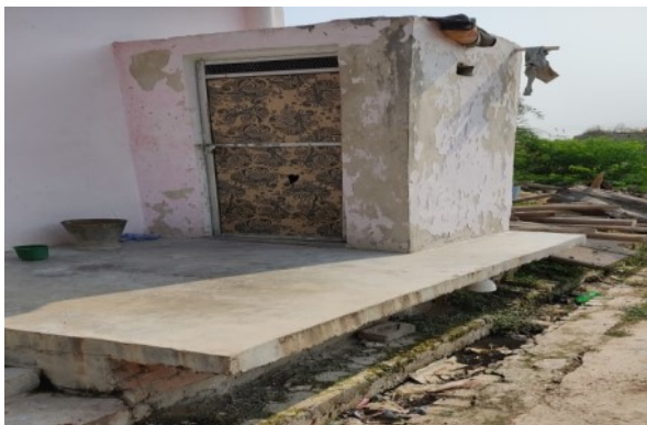
Figure 2: Toilet discharging directly to open drain.
