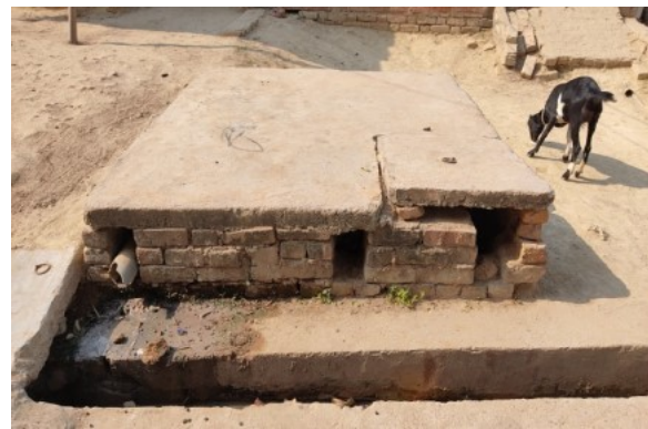
Figure 3: Lined tank with open bottom.
