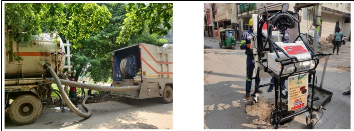
Figure 7: Cleaning of a sewer line in Sector 56 (left) and 'Robot' desludger used for cleaning small manholes (right). (Source: Uma/TRCSS, JNU (2021)).
