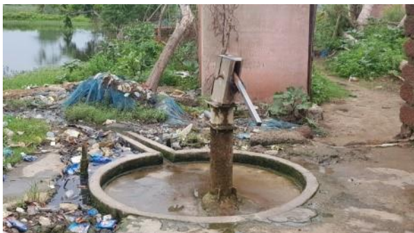
Photo 6: Drinking water source protection
