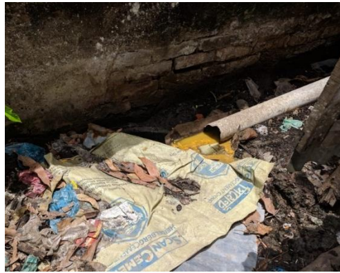
Right: Toilet pipe connected to open ground
