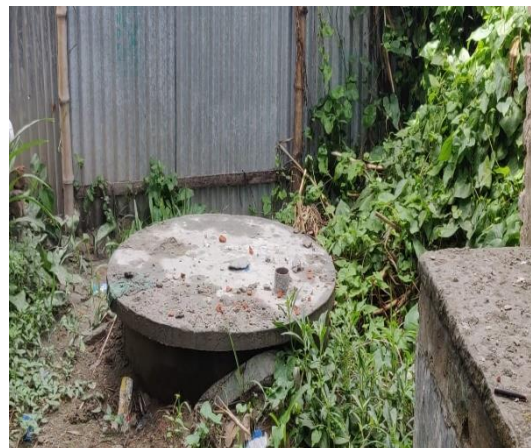
Right: Soak pit from septic tank
