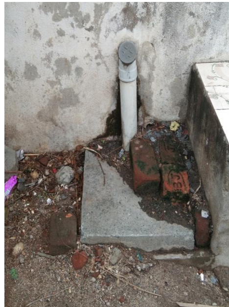
Figure 7: Septic tank outlet connected to soak pit (Source: Gowtham/CSE/2021)
