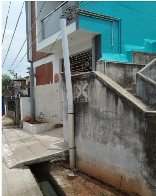
Figure 6: Septic tank outlet connected to open drain (Source: Gowtham/CSE/2021)
