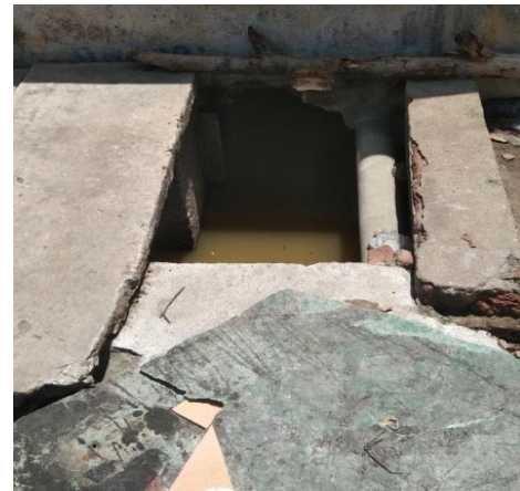
Figure 5: Sewer line in Kanchipuram Bus stand (Source: Gowtham/CSE/2021)
