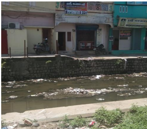
Figure 4: Effluent discharge pipe in manjal neer canal (Source: Gowtham/CSE/2021)
