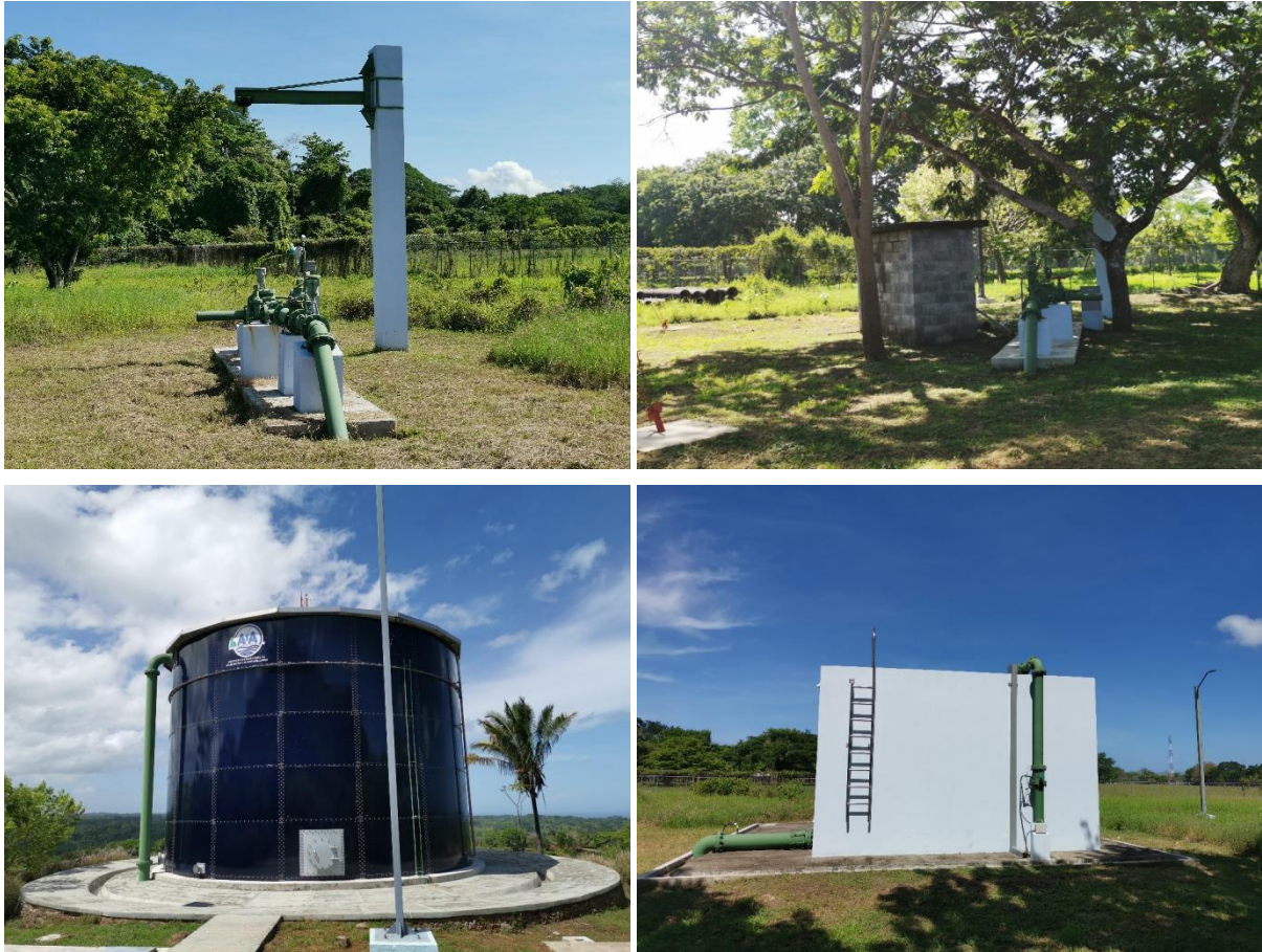
Figure 14: Arío - Santa Teresa - Malpaís Integral Aqueduct; (Above) Field of wells drilled in Bajos de Arío; (Below) Aqueduct deposits, located in Villalta and Santiago. Source: (AyA and PIIAG, 2015).
