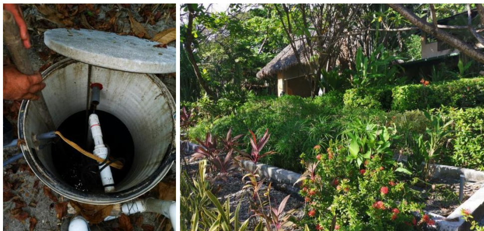
Figure 7: Privately-owned WWTP to treat wastewater and artificial wetland to treat greywater in a hotel in the area. Source: (Kenneth Alfaro Alvarado, 2021).
