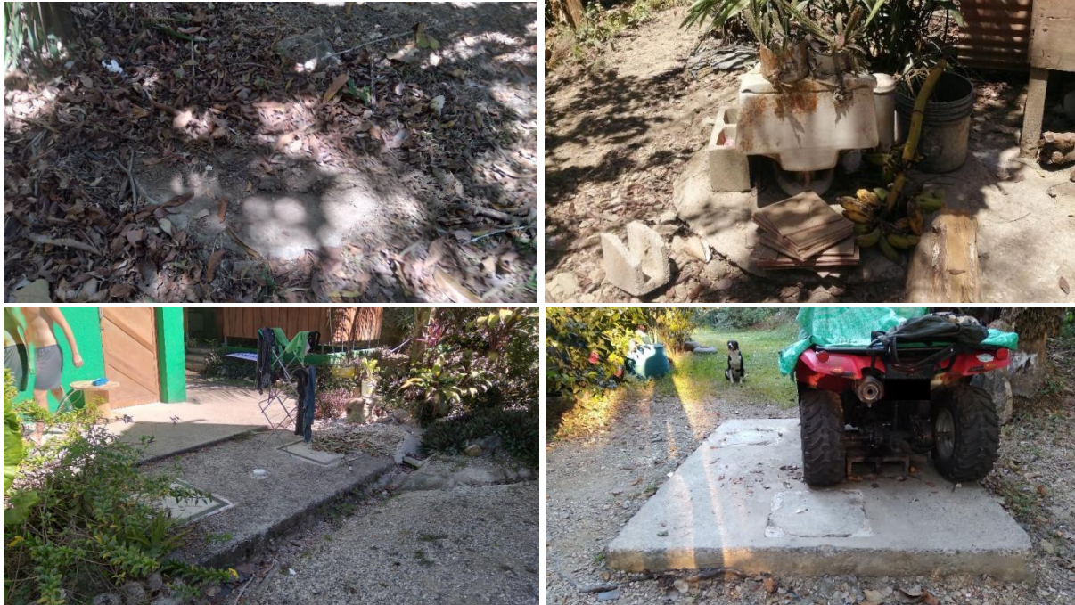
Figure 13: Above: Example of the soak pit of a lined tank with open bottom from a tourist place (left) and a household (right). Bottom: Example of a soak pit of a septic tank from a tourist place (left) and a household (right). Source: (IDB and WK, 2021a; IDB and WK, 2021b).
