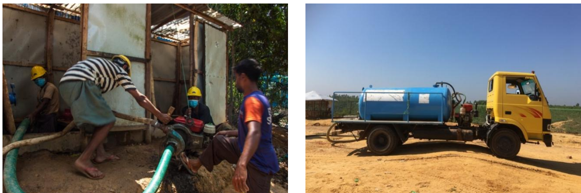
Figure 11: Left: Mechanical Emptying (Source: UPM, 2019) – Right: Vacuum Truck. (Source: UPM, 2019).
