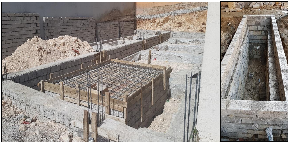
Figure 7: Typical holding tank arrangement in household construction. Permeable walls and no concrete slab in the base. (Source: Author, 2019)
