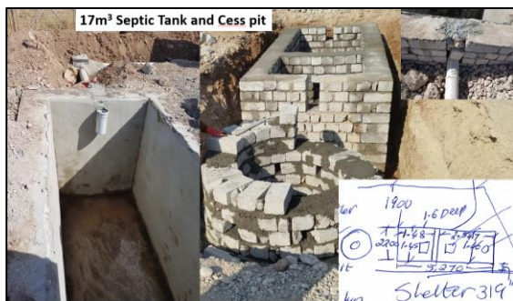
Figure 1: Recent Septic tank & soak pit design, Domiz 1. Similar construction in Domiz 2. (Source: Author, 2018)
