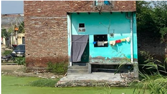
Figure 10: Septic tank connected to open ground, Zone 3 (Source: Urja Vashishth/CSE/2021).
