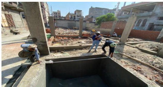
Figure 8: Fully lined tank with outlet In Zone 2, Jaitpur Village (Source: Sachin Sahani/CSE/2021).
