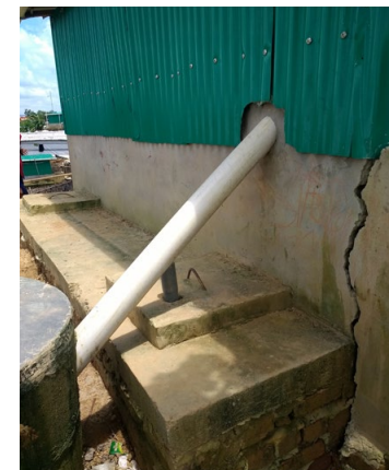
Example of latrine equipped with chute for discrete disposal of MHM material (PVC pipe connected to a sealed pit) (Source: IFRC/Swedish Red Cross)
