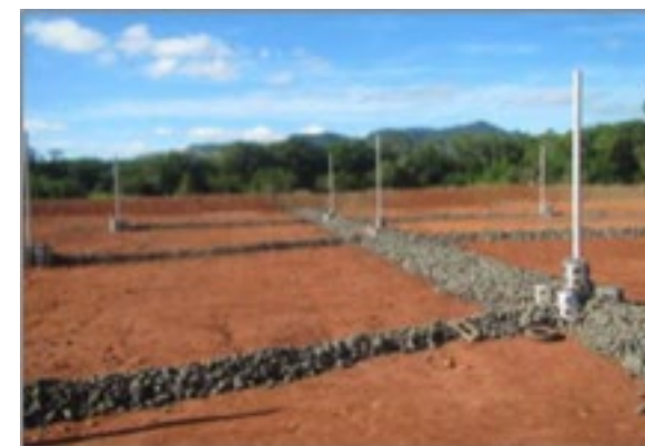
Key components of Fukuoka method – leachate collection and vertical gas venting pipes (Source: JICA/SPREP)
