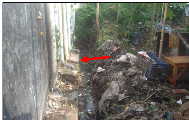
Toilet pipe connected to open drain
