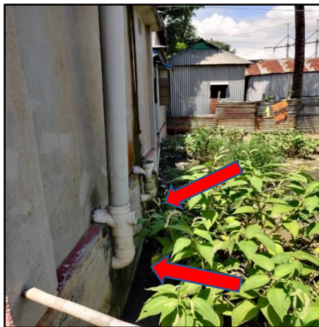
Left: Outlet connected to the uncovered drain
