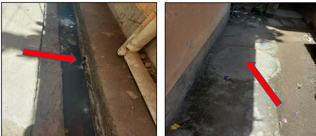
Figure 5: Left: Septic tank connected to a nearby drain. Right: Septic tank connected to soak pit. (Source: Field Survey, July 2021)
