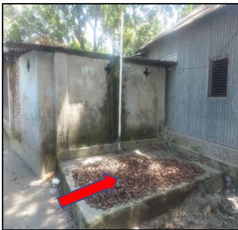
Left: Septic Tank
