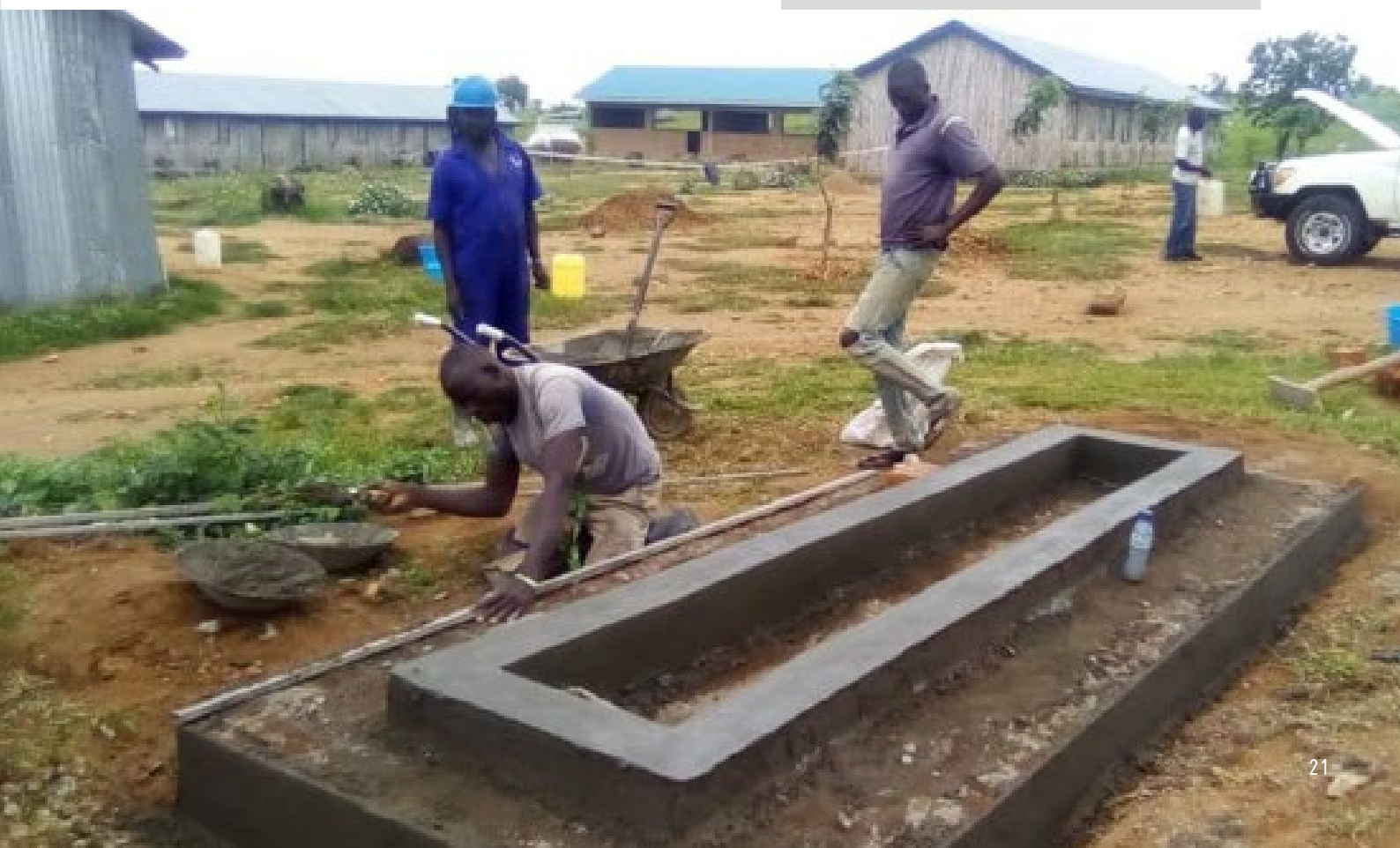
FIGURE 23 // WASHaLOT installed by Hand Pump Mechanic Association in West Nile (Source: WatSSUP, 2021)
