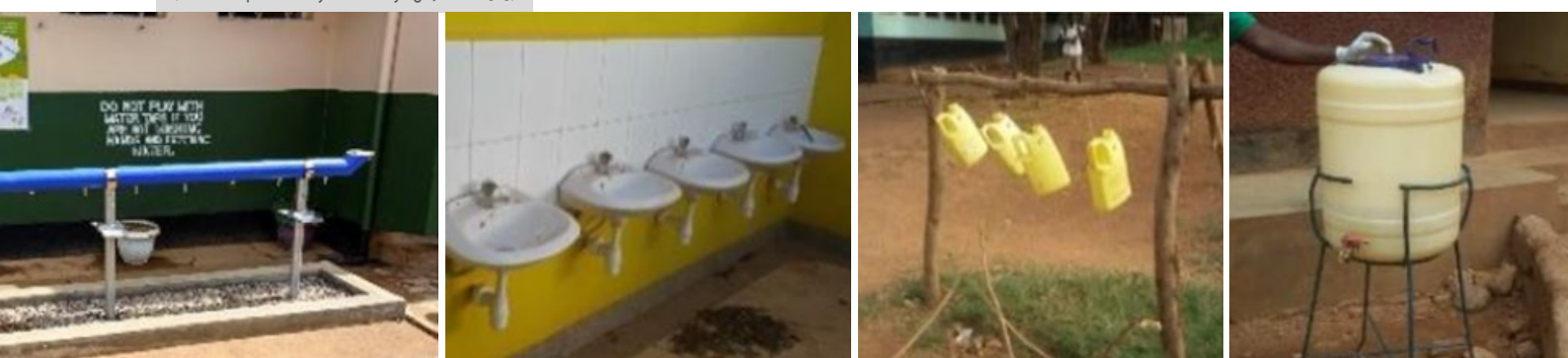
FIGURE 4 // WASHaLOT and conventional group handwashing facilities (Source: photos by S. Semiyaga, 2020 [7])
