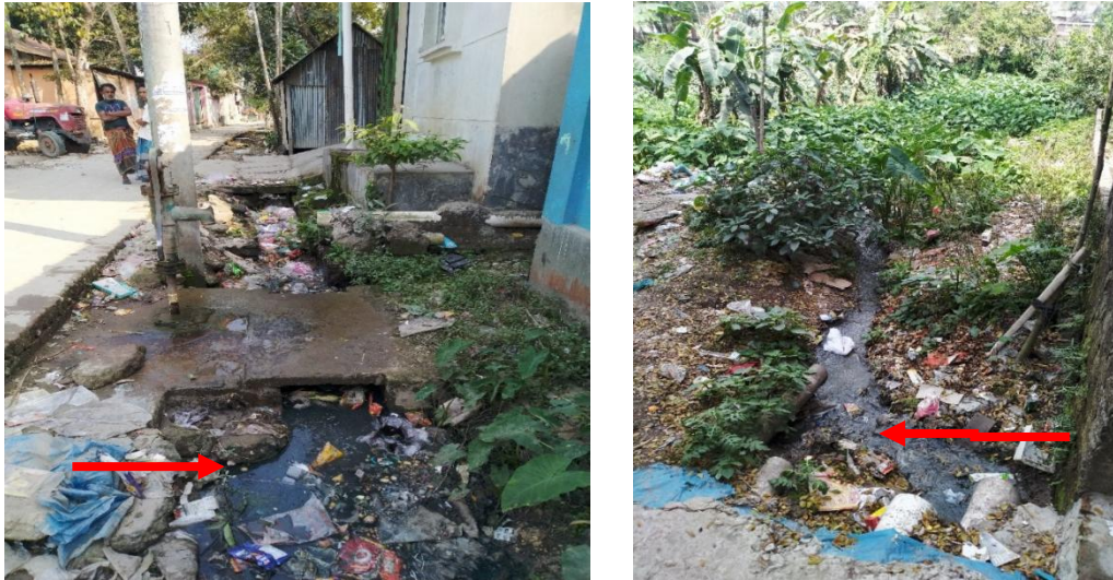
Figure 6: Containment technologies and their connections in Kishoreganj. Left: Septic tank connected to a nearby water body. Right: Toilet pipe connected to open drain. (Source: Feasibility study 2020-21/DPHE).
