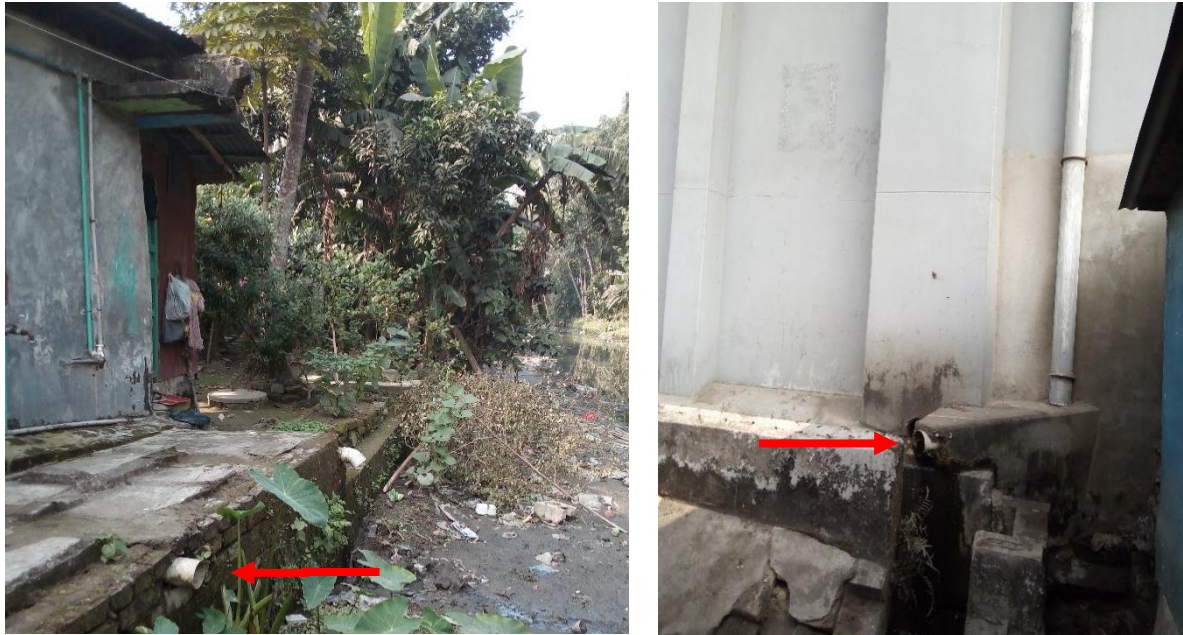
Figure 6: Containment technologies and their connections in Panchagarh. Left: Septic tank connected to the nearby water body. Right: Toilet pipe connected to open drain. (Source: Feasibility study 2020-21/DPHE).
