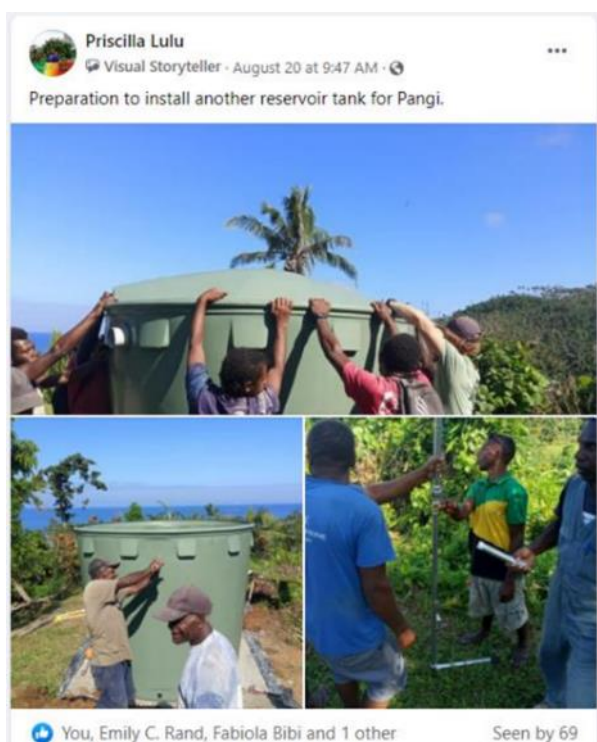
Figure 5: Monitoring infrastructure installations
