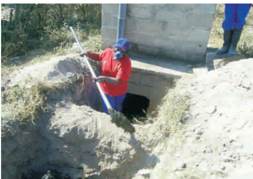
Figure 44a,b: Formalised pit emptying in eThekweni
