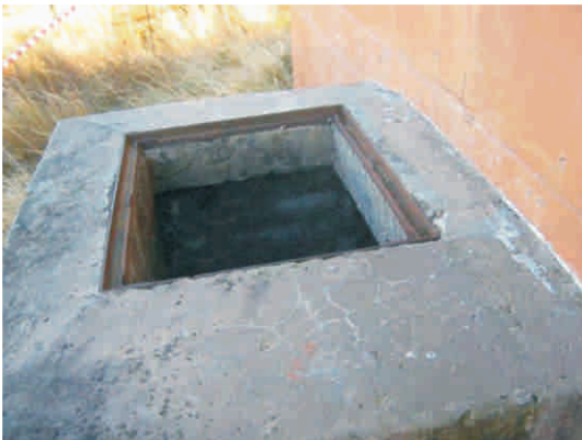
Figure 22 a,b,c: Toilet facilities in many schools are unusable due to poor maintenance, vandalism and inappropriate usage
