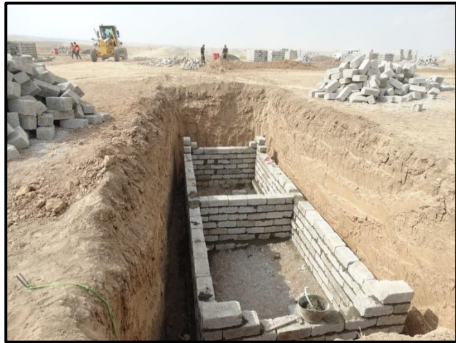
Figure 7 - Kabarto 2 Blackwater Containment, 1 of the total of 150. (Source: Duhok Governorate, 2021)
