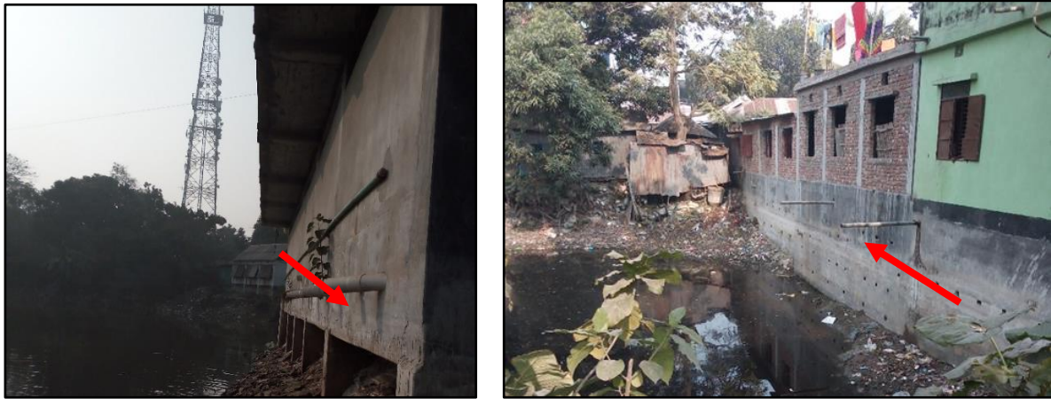
Figure 6: Containment technologies and their connections in Sirajganj. Left: Toilet pit open to a nearby water body, Right: Toilet pipe connected to open environment (Source: Feasibility study 2020-21/DPHE ).
