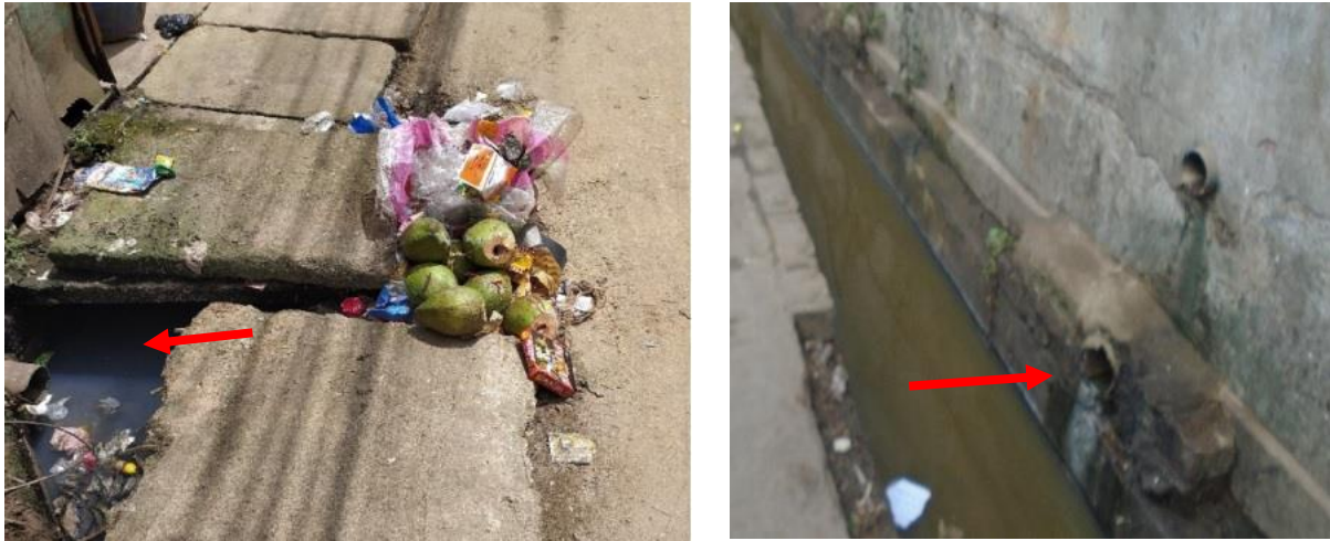
Figure 6: Containment technologies and their connections in Rajbari. Left: Septic tank connected to the nearby water body. Right: Toilet pipe connected to open drain (Source: Feasibility study 2020-21/DPHE).
