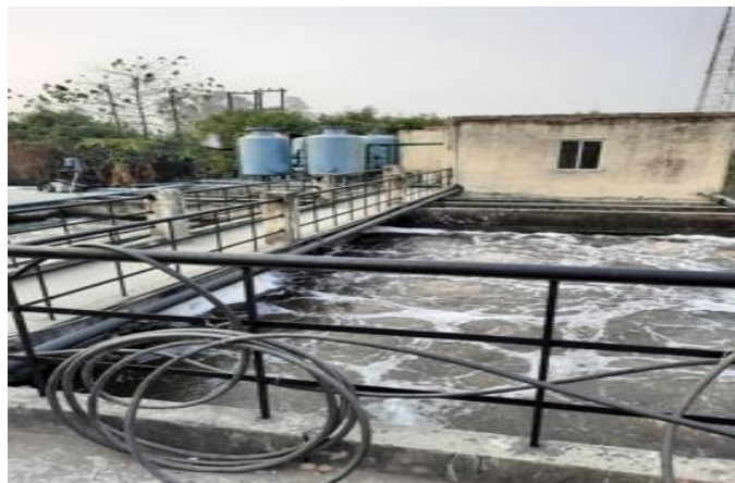
Figure 3. Sewage Treatment plant in Private Societies (Source: Aparna/NIUA/2021).
