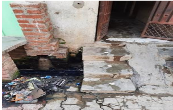
Figure 7: Fully lined tank connected to open drain (Source: Aparna/NIUA/ 2020).
