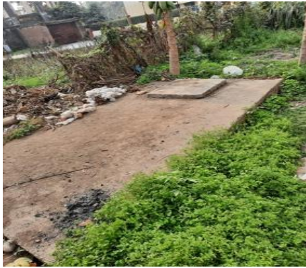
Figure 6: Septic tank connected to soak pit in ward no. 21 (Source: Aparna/NIUA/2021).
